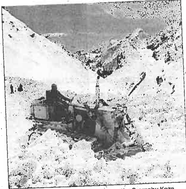
A snow-clearing operation underway on the Gramphu-Kaza highway in Lahaul-Spiti. TRIBUNE PHOTO
